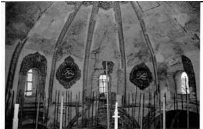
Figure 3. Cracks of the dome of the church Sergius and Bacchus.
