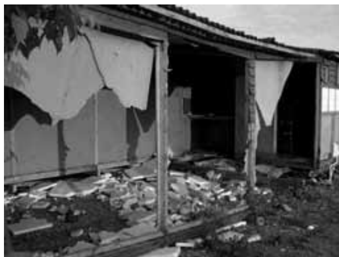
Figure 4. View of the temporary houses after evacuation.
