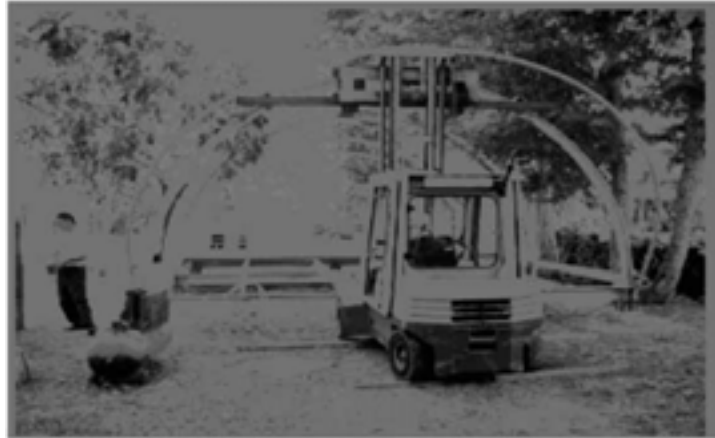
Figures 7-9. Horizontal load tests have been carried on the prototype by applying hydraulic jacks to the main frames and to the secondary structure.
