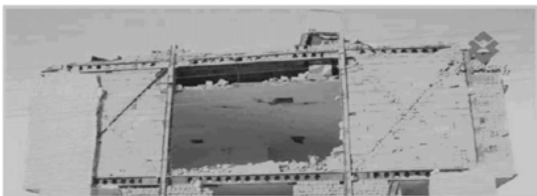
Figure 3. Fine-meshed steel structures in Bam 26-12-2003 (BHRC).
