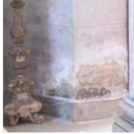
↑ Efflorescenze parete interna. Efflorescence on interior walls.
