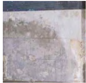
↑ Degradi pareti interne. Degradation of internal walls.
