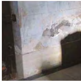
↑ Degradi intonaci interni. Degradation of interior plasterwork.
