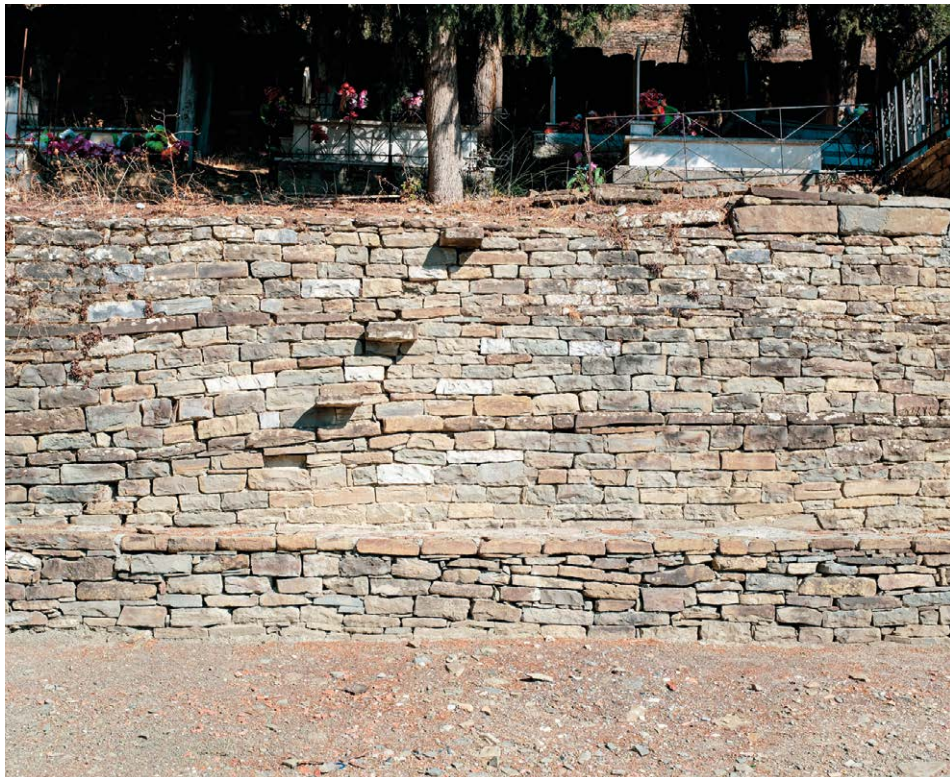
Figure 4.39 – The stone seat of the east parvis at the base of the cemetery retaining wall.
