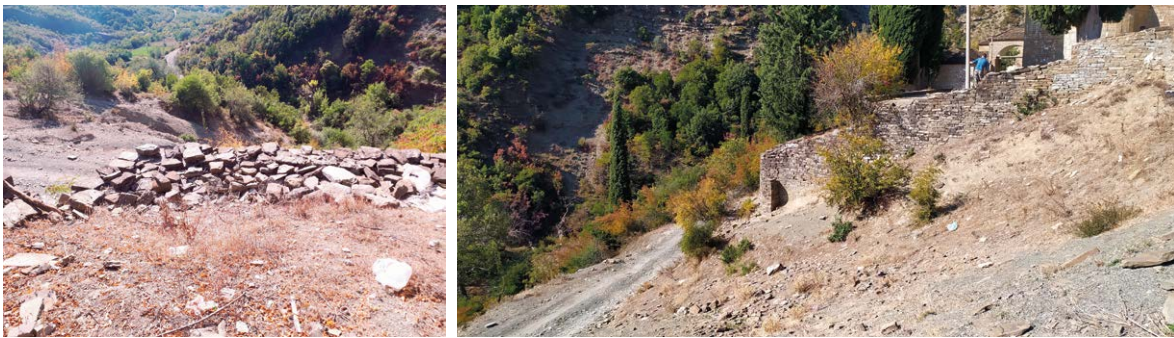
Figure 4.42 – State of deterioration of the walls supporting the terracings. Table 4.12 – Narrative master plan of Functional Lot 3: Interventions relating to the external areas adjacent to the architectural complex.
