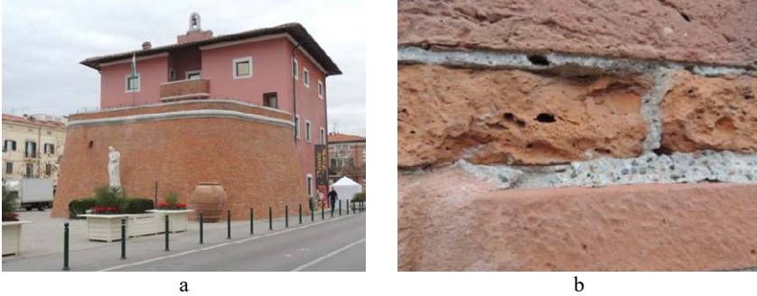
Figure 6 – Forte dei Marmi (a); particular of re-pointed mortar and brick erosion phenomena (b).
