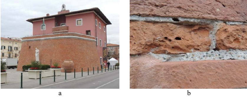
Figure 6 – Forte dei Marmi (a); particular of re-pointed mortar and brick erosion phenomena (b).
