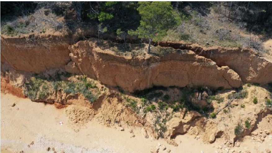
Figure 5 – Semi-detached part of the cliff with visible crack and root branches of Aleppo pine.
