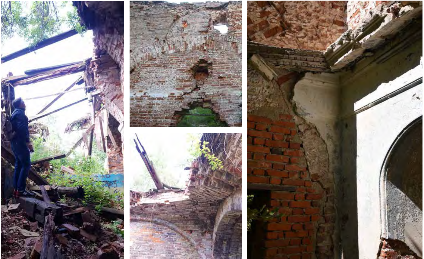
↕ Fig. 05 Restoration activities Interiors of the church of the Transfiguration of the Savior in Pyskor. On the right, details of the stratification of the brick wall and the plaster.
