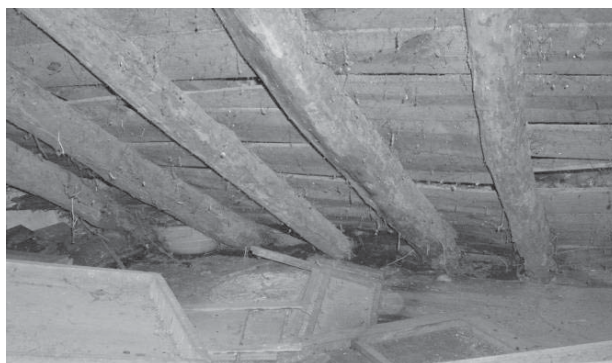
Fig. 4. Detail of the eucalyptus rafters showing destruction by wood rot and subterranean termites.
