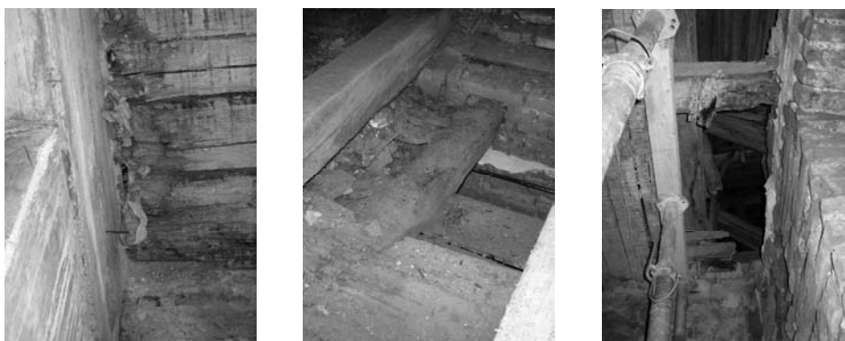
Fig. 10. Floors in the attics: brown rot on the supports, complete destruction of beams.
