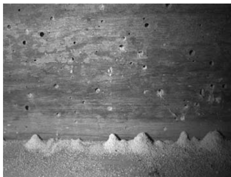
Fig. 12. Frass at construction
