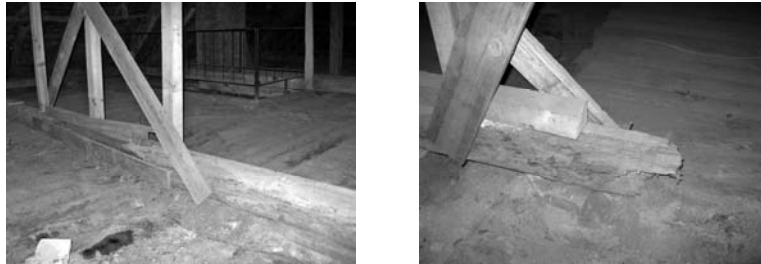
Fig. 7. Wood in the lower chord of the main frame and in the longitudinal tie beam completely destroyed.
