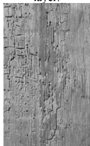
Fig. 7 – Damages by woodboring anobiid beetles.
