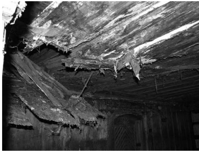
Fig. 4 Vault decayed by the Coniophora puteana and other fungi
