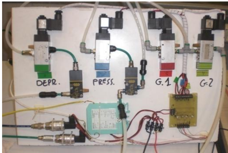
Figure 7 – Panel with the electro-valves, transducers and driver
