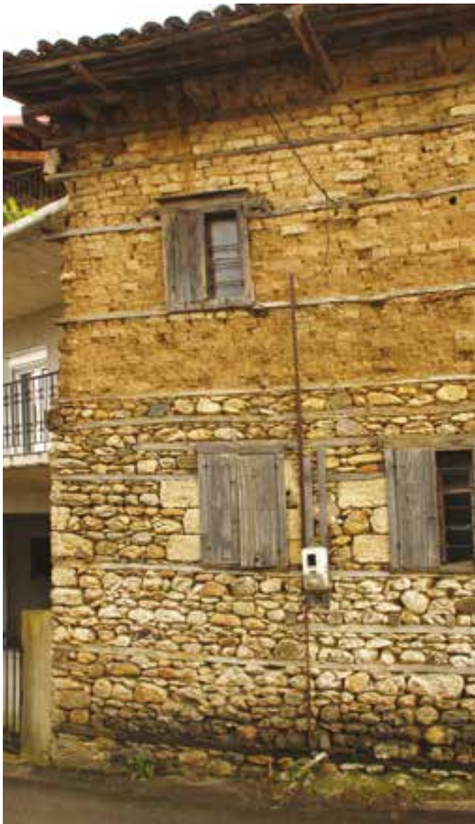
Fig. 13 Stone and adobe building with hooping reinforcement in Kastaneri, Greece (photo: S. Mecca).
