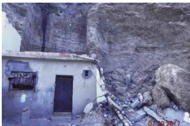
Photo 4 – Crumbling dune cliffs shattered by the action of the sea, causing the destruction of fishing shelters and houses that encroach into the sea at Bousfer beach. (Credit photo: A. Bougherira).
