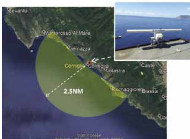
Figure 6 – X-band coastal radar installed in Corniglia.
