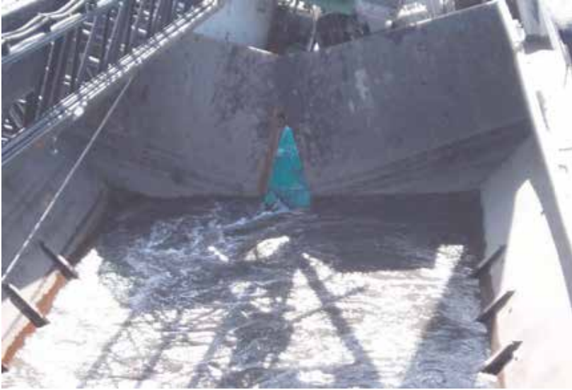
Figure 5 - Opening which enable the water to fill the housing for the clods.
