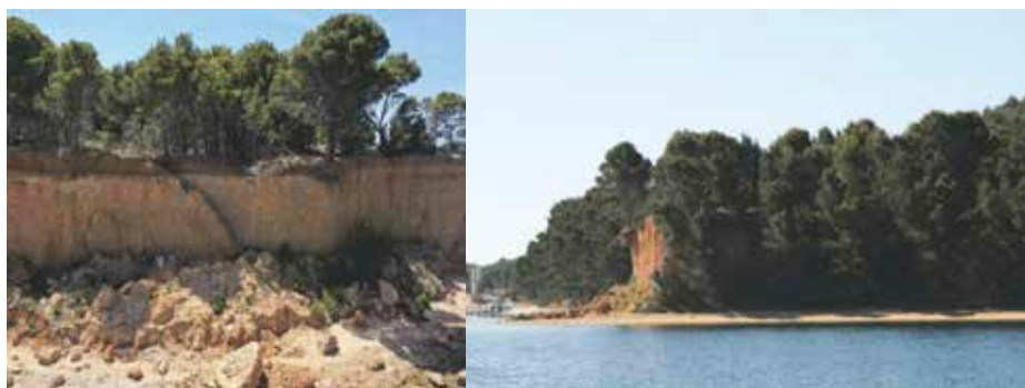
Figure 2 - Eroding coastal cliff on the Vrgada Island; view from east (left photo) and from north (right photo).
