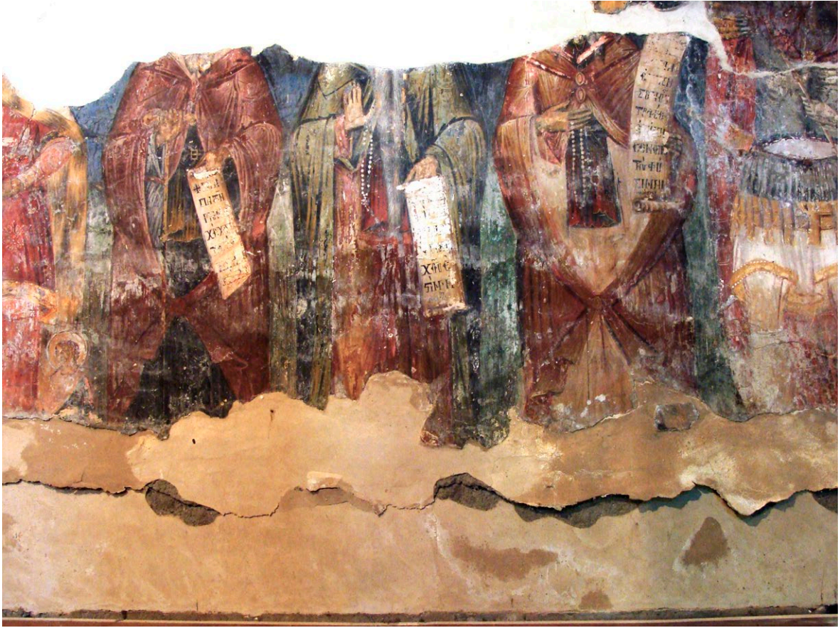
Figure I-5.3.11 Severe damage on the south wall of the church due to the rising damp.
