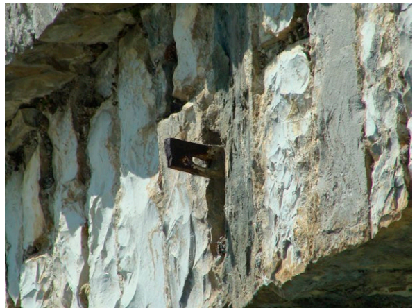
Figure I-5.1.5 – A detail of the head of a transverse steel tie rods lacking of wedge.
